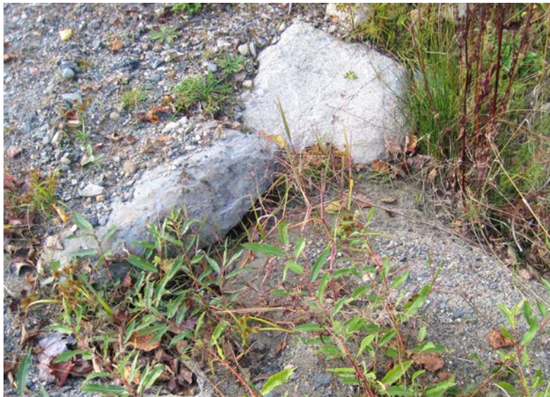
Blocked culvert in North Country Region
