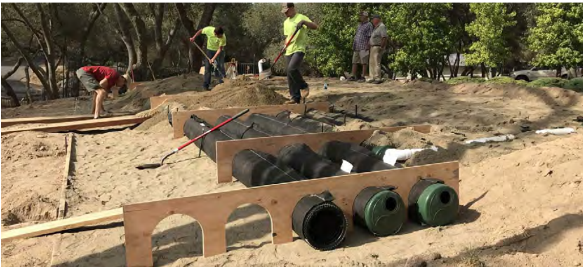
Installation of the municipally owned Blodgett Landing community septic system in Newbury. (Images via NextGen Septics)
