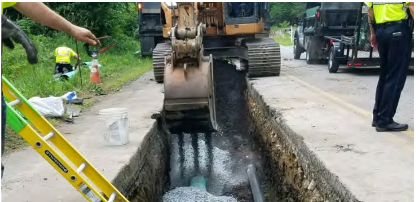
Sewer construction in the Five Corners growth area in Easton, MA, funded in part through Tax Increment Financing. Once complete, the new sewer capacity will allow more housing development and absorb growth from more rural areas of town. (Image via Town of Easton, MA.)
