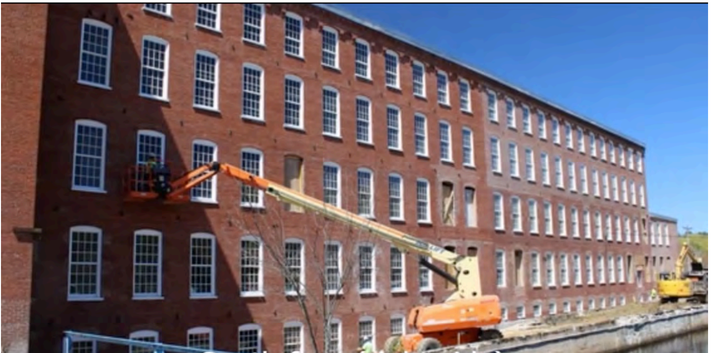
Construction underway at the China Mill rehabilitation project using 79-E in Allenstown, NH. (Image via allenstown-alt.com )
